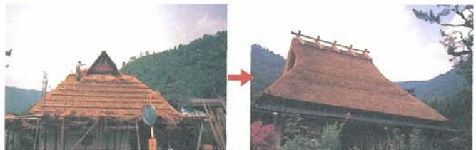
Repair of a historic building (vernacular house with thatched roof) at Kita, Miyama-cho
