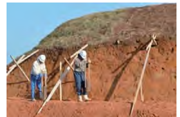
Photo 4-3 Repair work on the burial mound slope at Tomb 25 after it collapsed, at the Shimbaru-Nuyama Mounded Tomb Group (2014)
